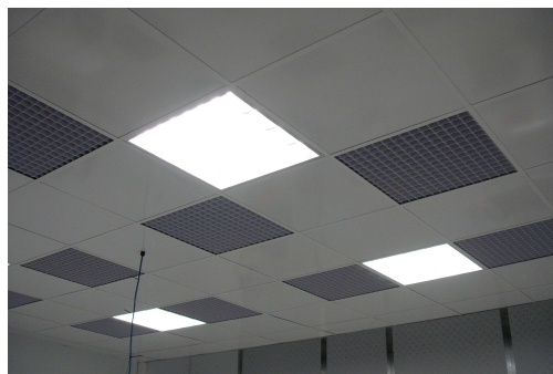
False ceiling with air outlets
