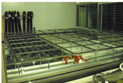
Hydraulic pipeworks in raised floor
